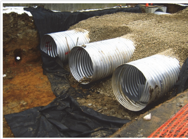
Source: Abington Township The township decided to use the property on Hamel Avenue as an underground stormwater detention area. In 2007, the township used capital improvement funds to construct a series of pipes in a stone bed for this purpose. After construction, the township replanted grass to make the area look like open space.
