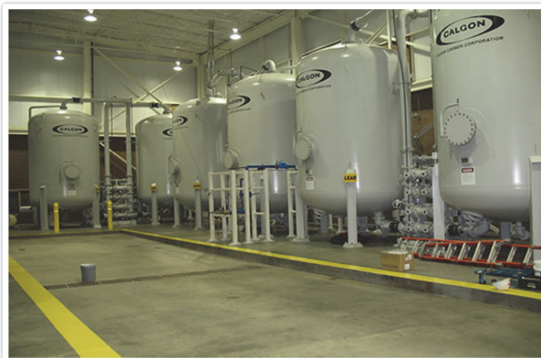
Source: Warrington Township A series of granular activated carbon filtration tanks used to treat contaminated groundwater in Warrington Township.
