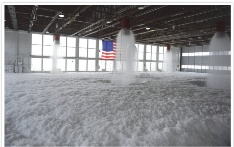
Source: Warrington Township This photo shows a system that is distributing fire-fighting foam in a military hangar.
