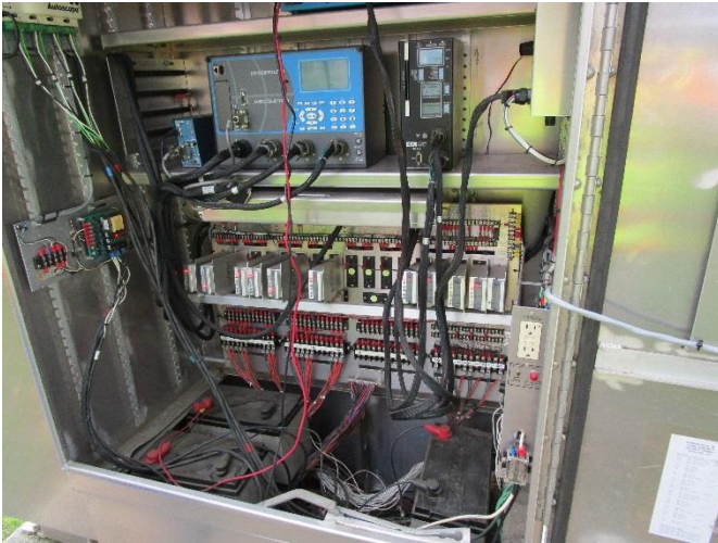
Photo 2: NEMA TS-1 controller (Econolite ASC/3S) at Prospect Street
