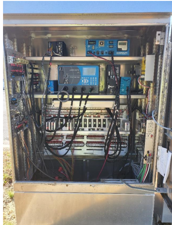
Photo 2: Controller Assembly at S. Mill Road
