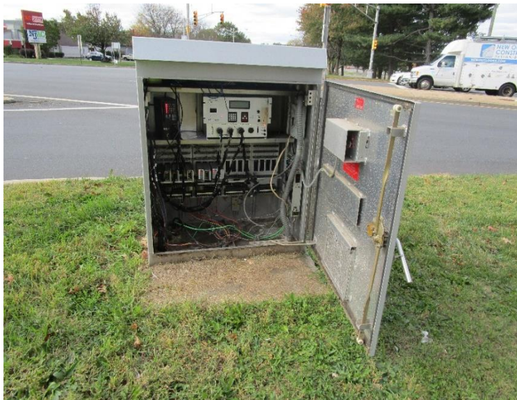
Photo 5: Controller cabinet at Quakerbridge Road and Clarksville Road (May, 2019).
