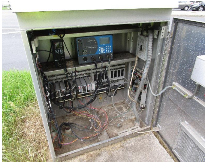
Photo 4: Controller cabinet at Quakerbridge Road and Clarksville Road, November 2018
