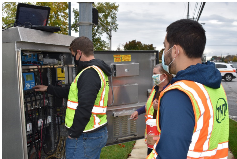
Photo 5: Left to Right: Brian Jatzke, Iteris; Colleen Richwall, Corridor Project Manager, TWT; and Dan Miller, TWT install new timings at Town Center Drive.
