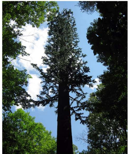
Cell towers can be designed to mimic trees and blend in with their surroundings.
