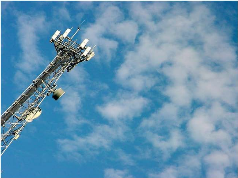
A typical wireless service facility, or “cell tower.”
