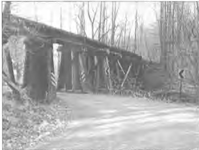
This timber-constructed bridge of the former Pomeroy & Newark RR has held up well over the years. Efforts should be put in place to preserve these historic resources and protect them from decay, vandalism and destruction. East Fallowfield/Highland Twps., Chester County.
