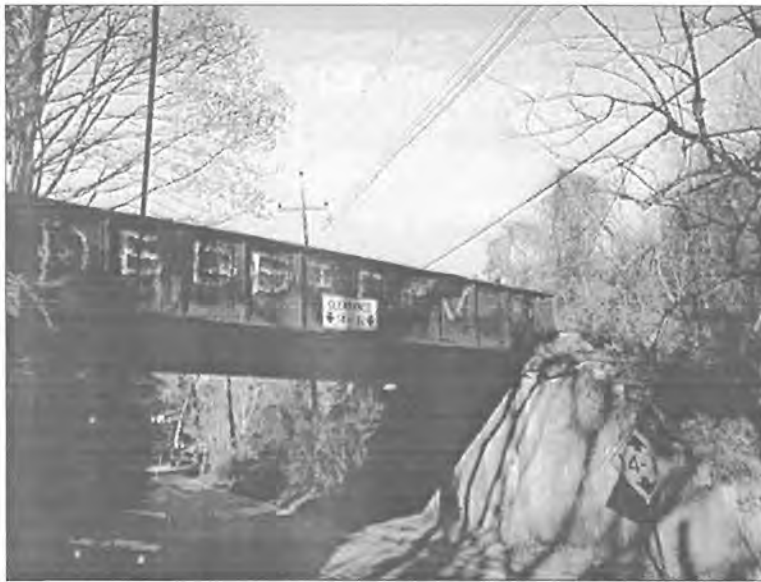
A bridge from the former Philadelphia & Western (P&W) which will be utilized in the Radnor Township Bike Path. (Radnor Twp., Delaware County)
