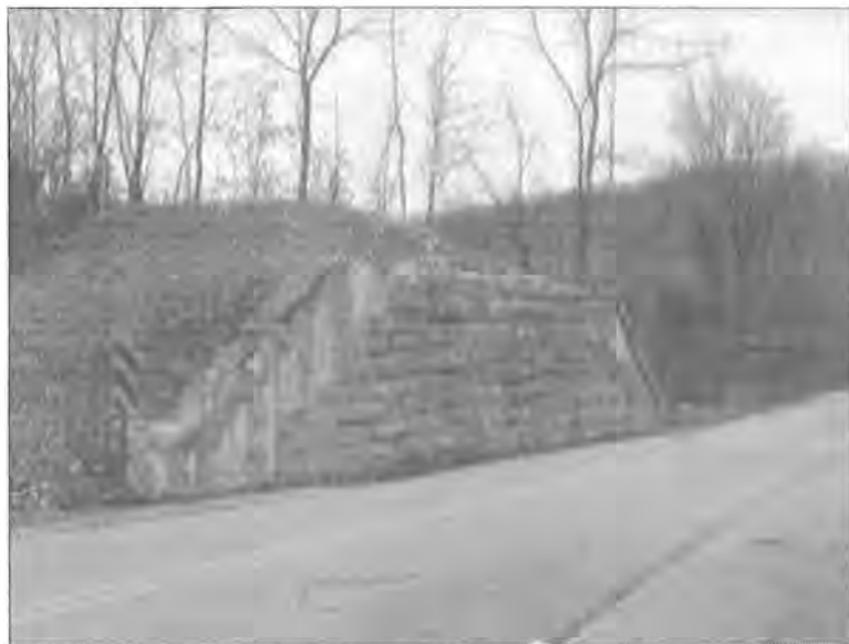
This is a typical scene of former overhead crossing. The grading and most of the stone abutment are still intact, but the bridge structure has been removed. Across the street, the abutment and RR grade were demolished for an access driveway to a new office complex. (Former Perkiomen Branch, just north of Rt. 422 in Upper Providence Twp., Montgomery County)
