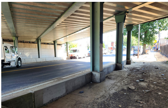
Crossing between distant crosswalks ( first image ); truck traffic approaching crosswalk ( second image ); and debris below underpass during the field audit ( third image )
