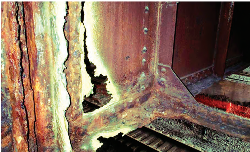
Example of bridge corrosion. Source: PennDOT.
