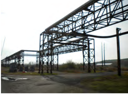
Some of the utilities at the Keystone Industrial Port Complex (KIPC) in Falls Township, Bucks County.
