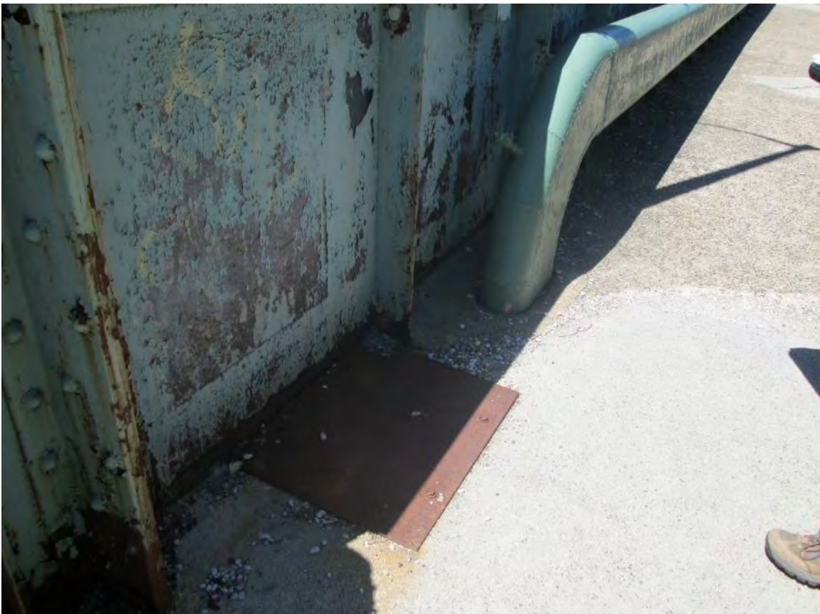
Figure 36 – Existing Plate on Sidewalk
