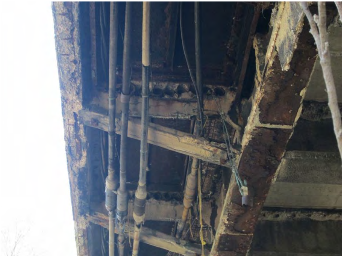
Figure 2 – Underside of sidewalk, showing 10 existing conduits
