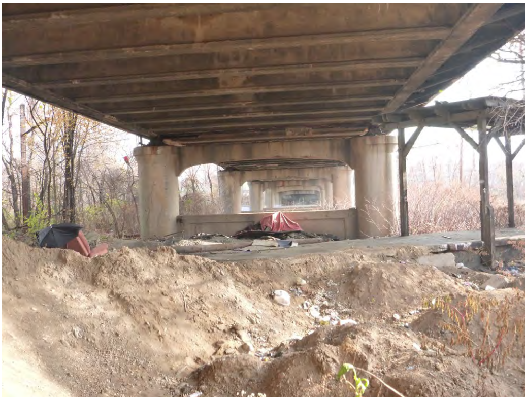
Plate 8: Lincoln Avenue Bridge, beneath bridge, detail of the girder span and stringers.
