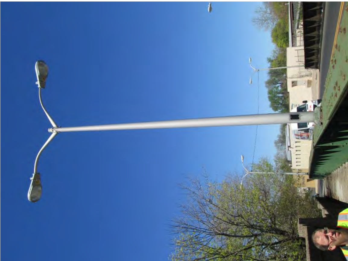
Figure 54 – Existing Light Fixture on Bridge (Typical)
