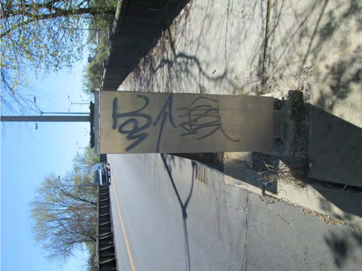
Figure 55 – Existing Meter Cabinet along Lincoln Avenue near Creekview Drive
