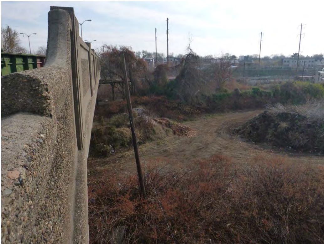
Plate 12: Lincoln Avenue Bridge, west parapet with debris pile west of bridge.
