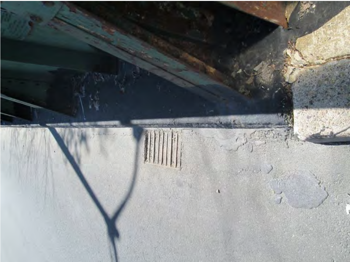
Figure 56 – Existing Blocked Drainage on Bridge (Typical)
