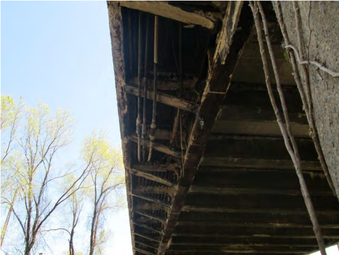
Figure 3 – Underside of sidewalk, showing 10 existing conduits
