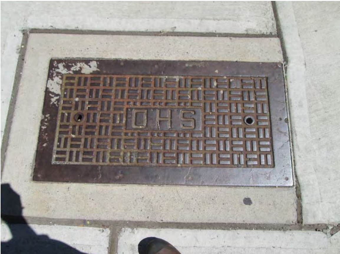
Figure 44 – Southwest quadrant of Lincoln Avenue and E. State Street, showing junction box
