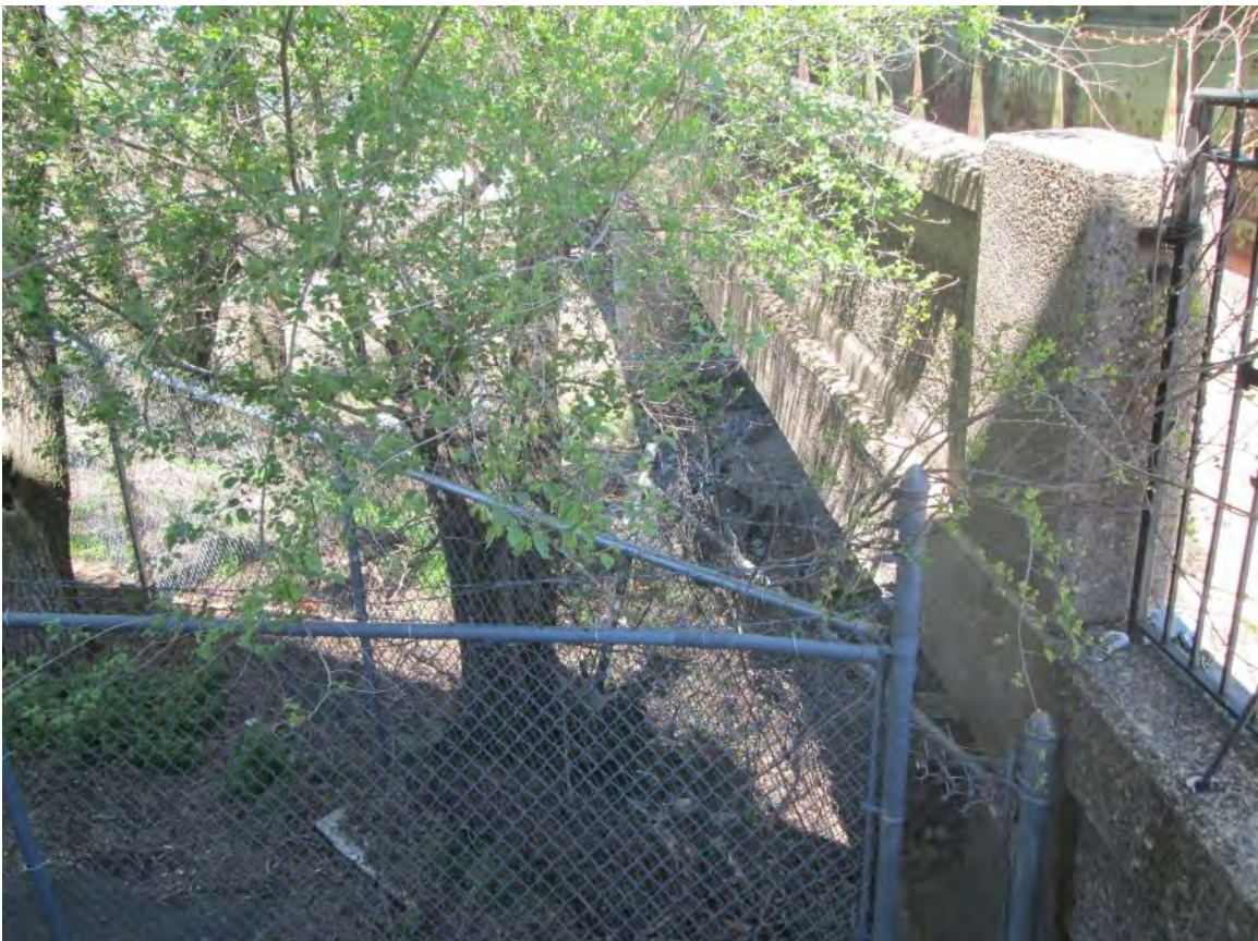
Figure 50 – South Side of Bridge, looking west at existing fencing behind CYO E. State Street Center
