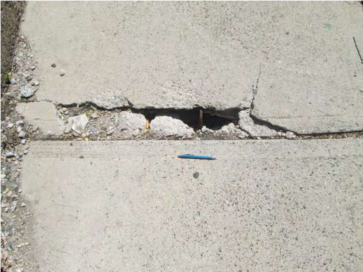
Figure 33 – Missing Sidewalk and Exposed Rebar (Typical)
