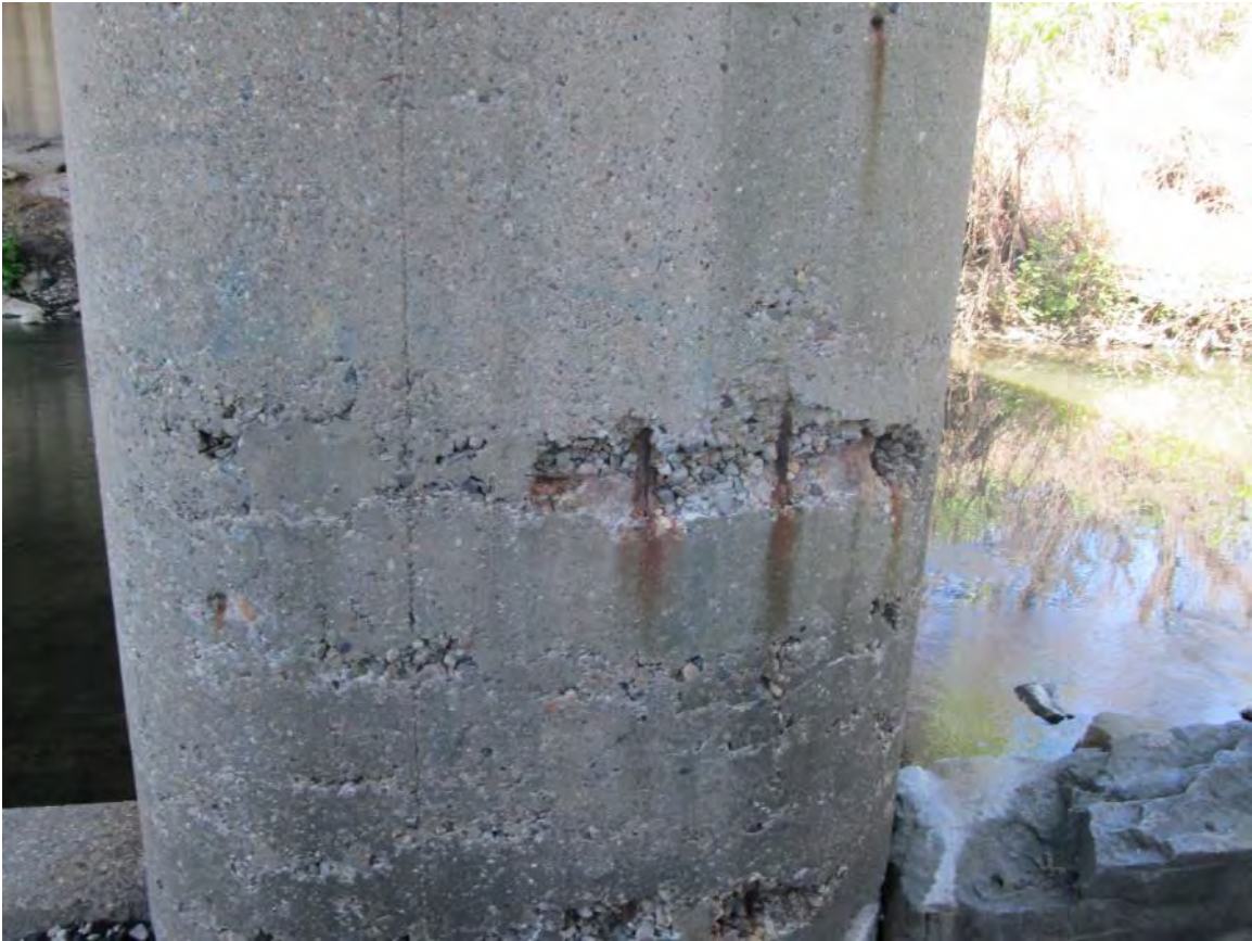
Figure 15 – Pier 7, showing concrete condition and exposed rebar
