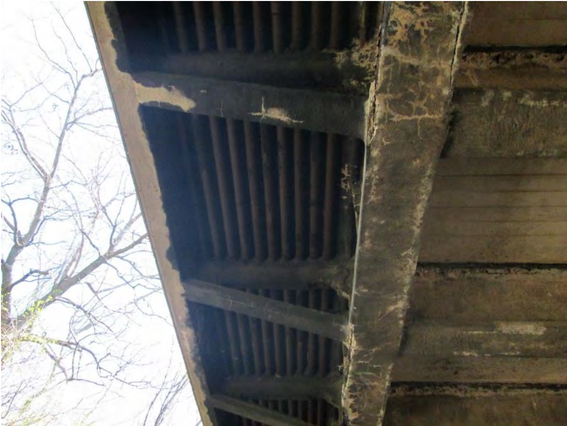
Figure 11 – Underside of sidewalk, showing 10 existing conduits
