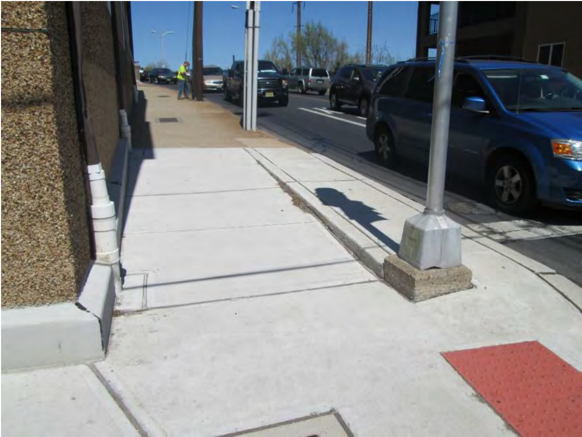
Figure 45 – Southwest quadrant of Lincoln Avenue and E. State Street, looking northwest showing sidewalk
