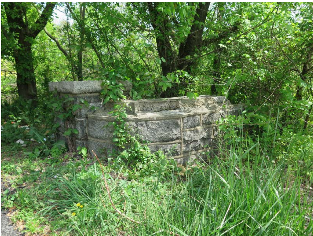
Plate 16: Remnants of a stone staircase adjacent to the Kaighns Avenue Bridge.
