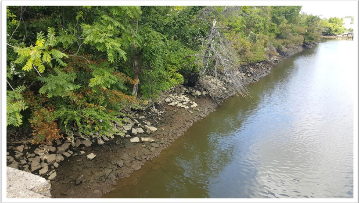
Photo A: View, facing northwest, of the west bank of the Cooper River, to the north of Kaighn Avenue Bridge.
