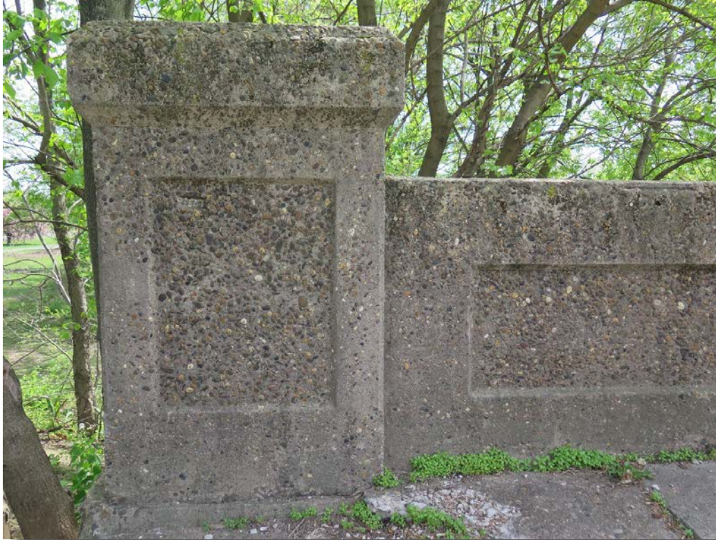
Plate 11: Detail of parapet on the southern span of the Kaighns Avenue Bridge.
