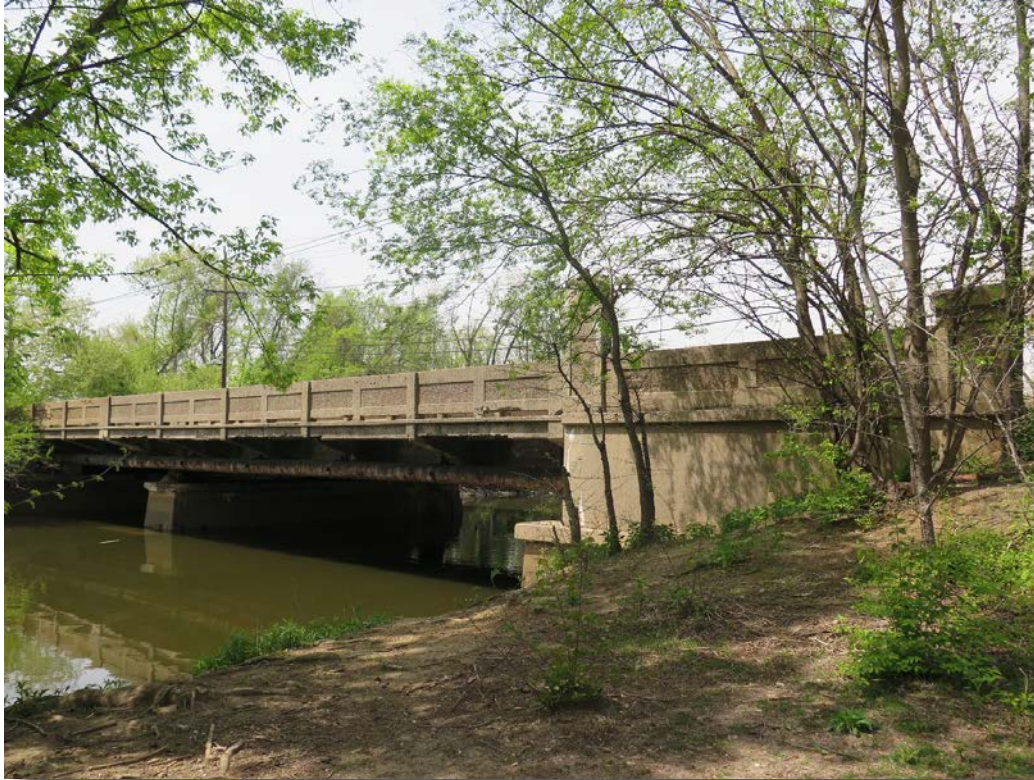
Plate 9: View northwest of the southern span, piers and undergrade of the Kaighns Avenue Bridge.
