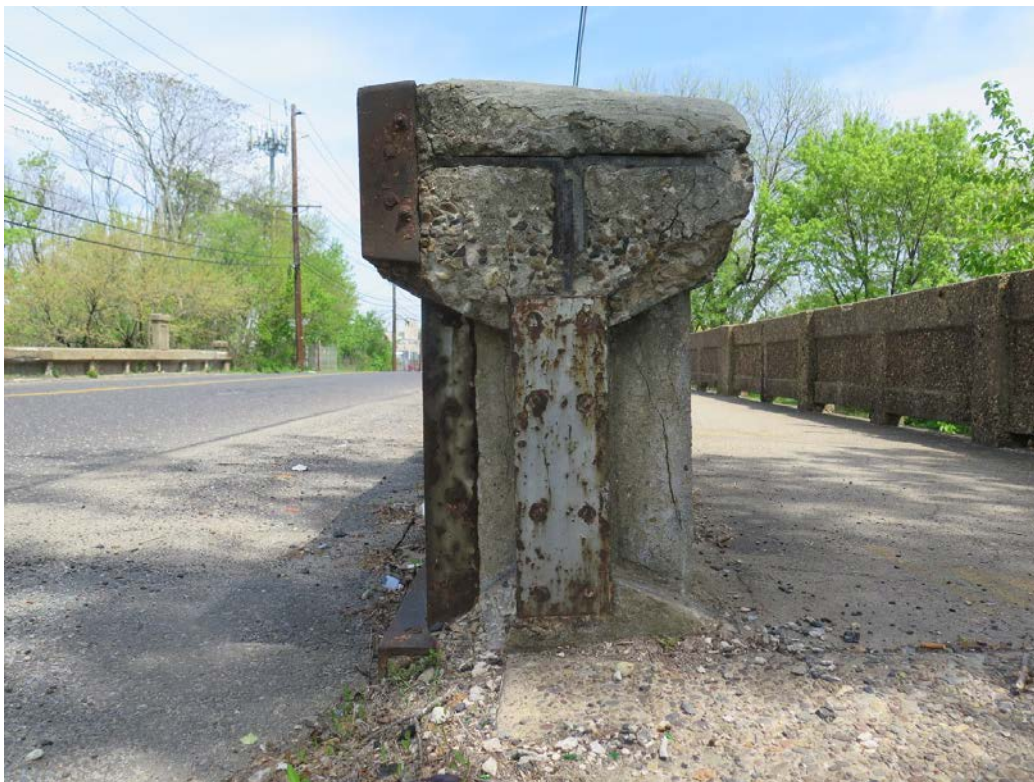
Plate 12: Detail of an iron T-bar underneath spalled concrete on the pedestrian barrier on the southern span of the Kaighns Avenue Bridge.
