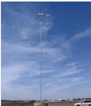
Guyed Monopole Tower
