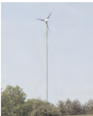
Windward Engineering Endurance 4.25kW turbine in Arkport, NY
