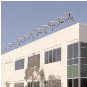
AeroVironment rooftop array
