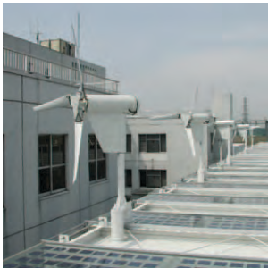
Proven Energy 2.5kW turbine rooftop array
