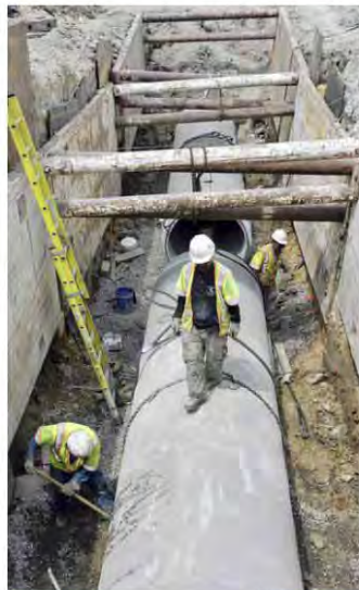
Baltimore Water Pipe
