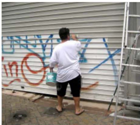
Removal of graffiti is an important maintenance step in maintaining the perception of safety. Source: Vibrant Streets, Washington D.C.
