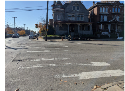
Faded crosswalks, like this one at Hunting Park Avenue and Old York Road, detract from pedestrian safety.
