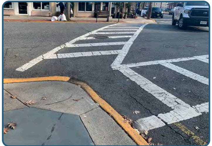
Some curb ramps at-- major intersections are not ADA compliant.
