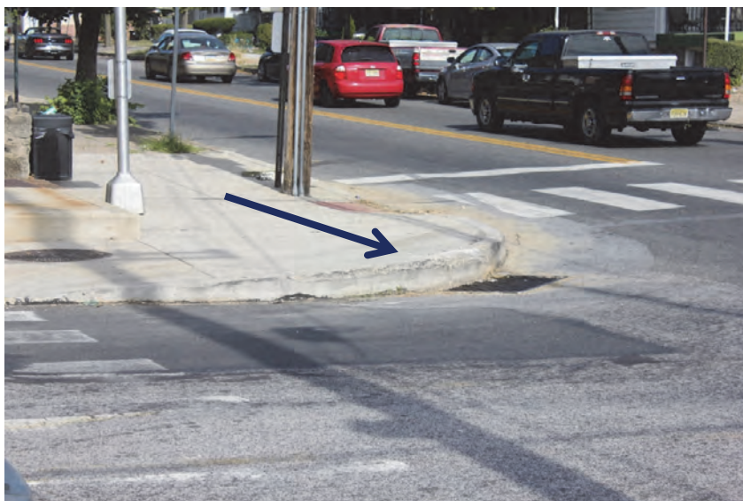
A damaged curb at Engle Street and 9th Street/US 13. Some intersections in the City of Chester were not designed to accommodate large trucks, which require wide turning radii. When trucks attempt these tight turns, they can overrun the curb, damaging the sidewalk and endangering pedestrians. Source: DVRPC, 2017
