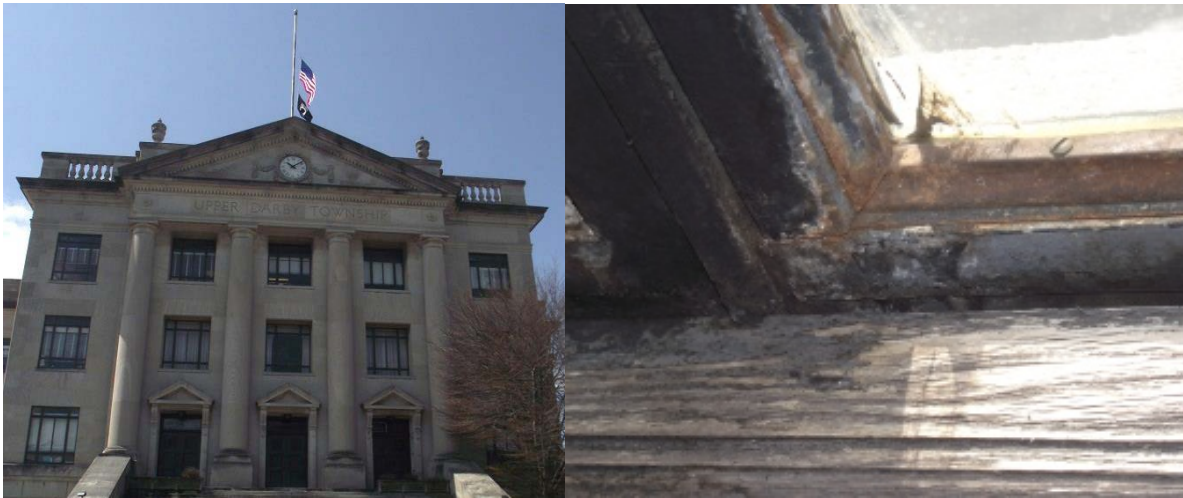
Figure 6: Original Windows, Frame Damage
