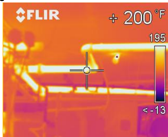
Figure 4: Heat Loss via Uninsulated Steam Pipes
