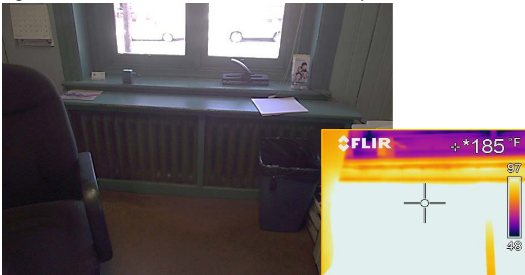
Figure 3: Uncontrolled Steam Radiator in Close Proximity to Office Worker's Desk
