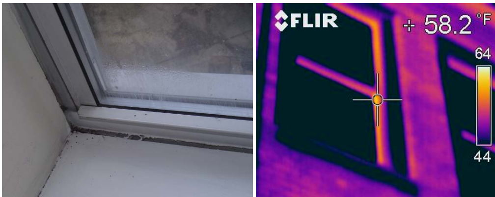
Figure 5: Insufficient Window Frame Sealing (L), Exterior Infrared Photo Showing Heat Escape (R)
