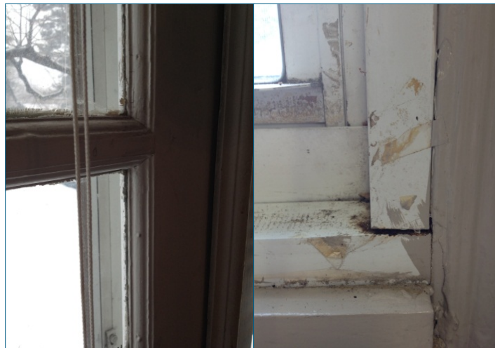
Figure 3: Window Frame Damage
