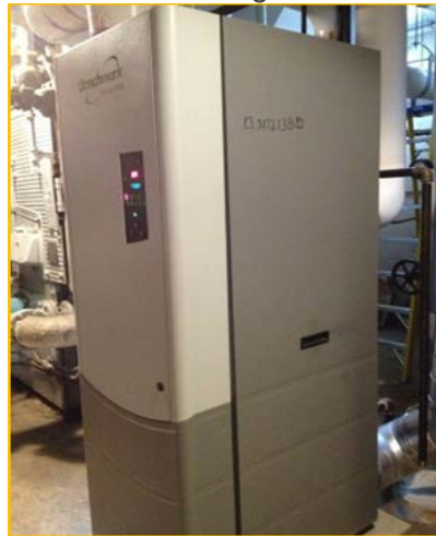
Figure 5: Condensing Hot Water Boiler
