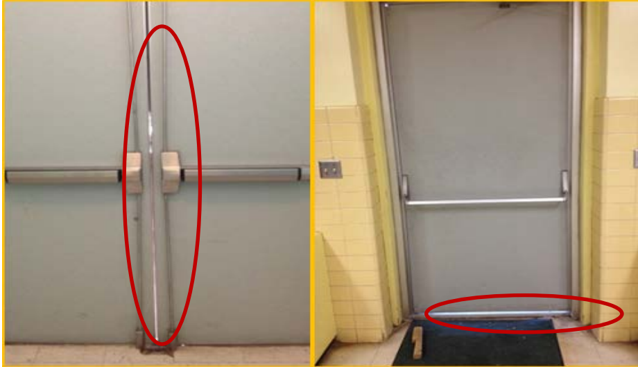
Figure 9: Doors Lacking Weatherproofing/Sweeps
