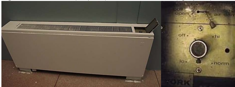
Figure 5: Fan Coil Unit (left photo) with Manual Controls (right photo)
