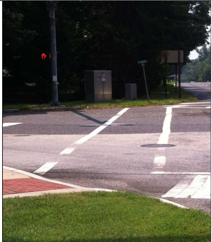
Faded crosswalk and missing curb ramp (far side)
