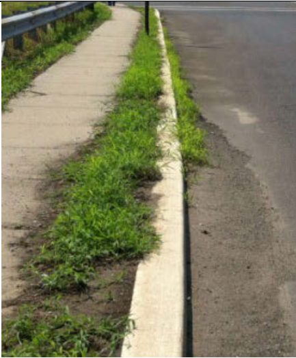
Debris from ponding along the curb in the northbound lane
