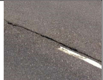
Roadway pavement cracking in several locations
