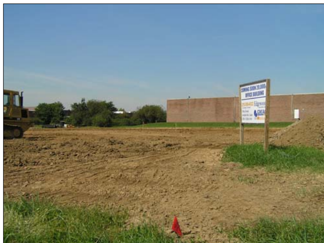
Office development infill in the Newtown Commons Business Park Photo by: DVRPC
