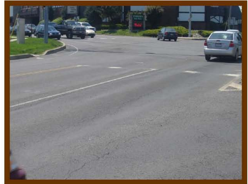
Faded pavement markings at the Hulmeville Road intersection
