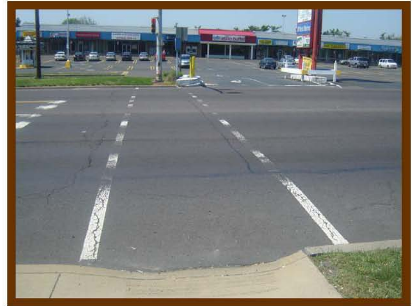
Pavement marking faded at Bensalem Plaza. Pedestrian signal head needs upgrading to man/hand with countdown timers
