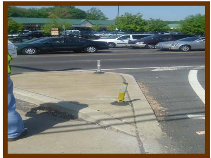
Delineators for right turn channelized island are damaged, intersection of Mechanicsville Road
