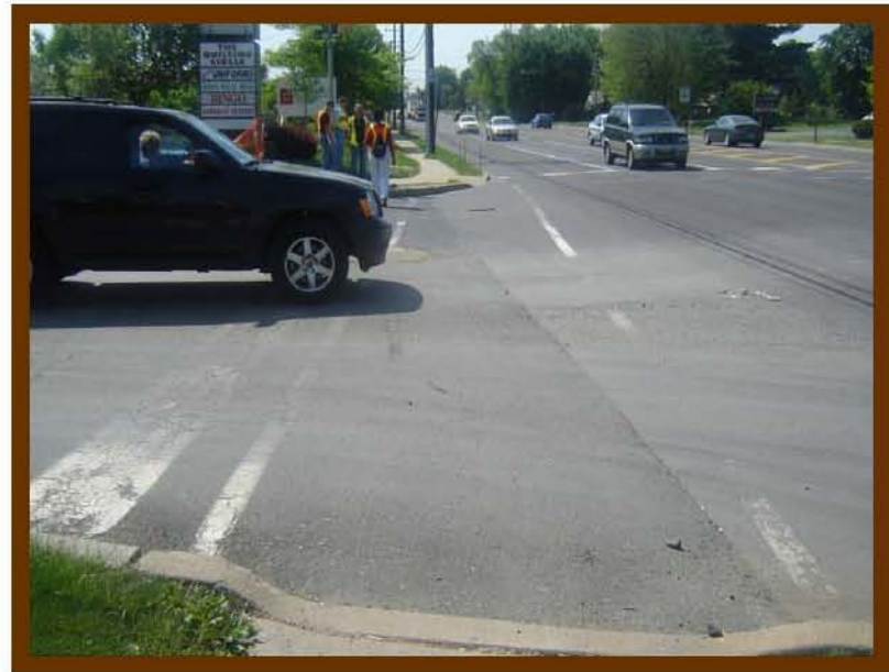
Faded pavement markings on Street Road and the shopping center driveway west of Castle Drive.
