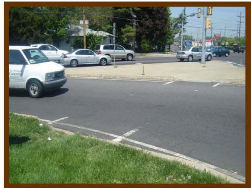
Pavement markings faded. Crosswalk and curb ramp lead to grassy area
