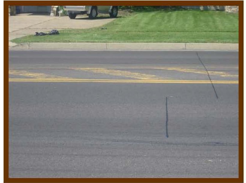
Faded pavement markings
