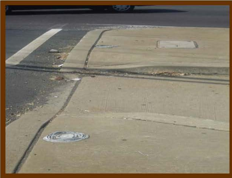
Delineators for right turn channelized island have been destroyed, intersection of Mechanicsville Road
