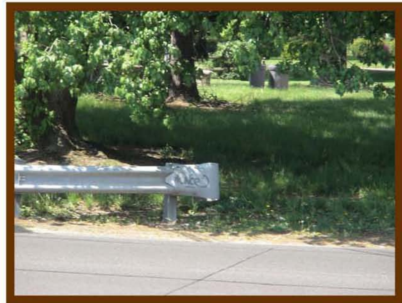
Guide rail with obsolete end treatment
