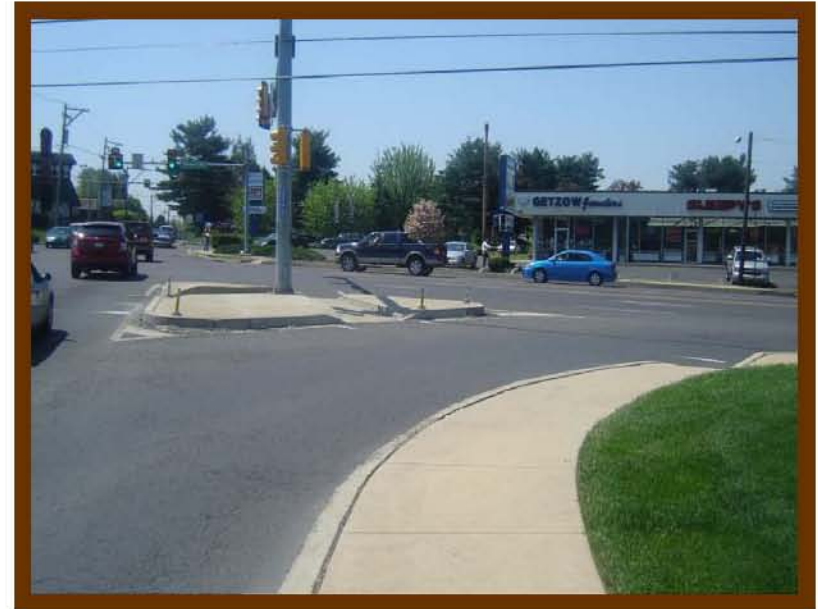
Pavement marking faded and no "yield" sign at the channelized right turn at the Hulmeville Road intersection
