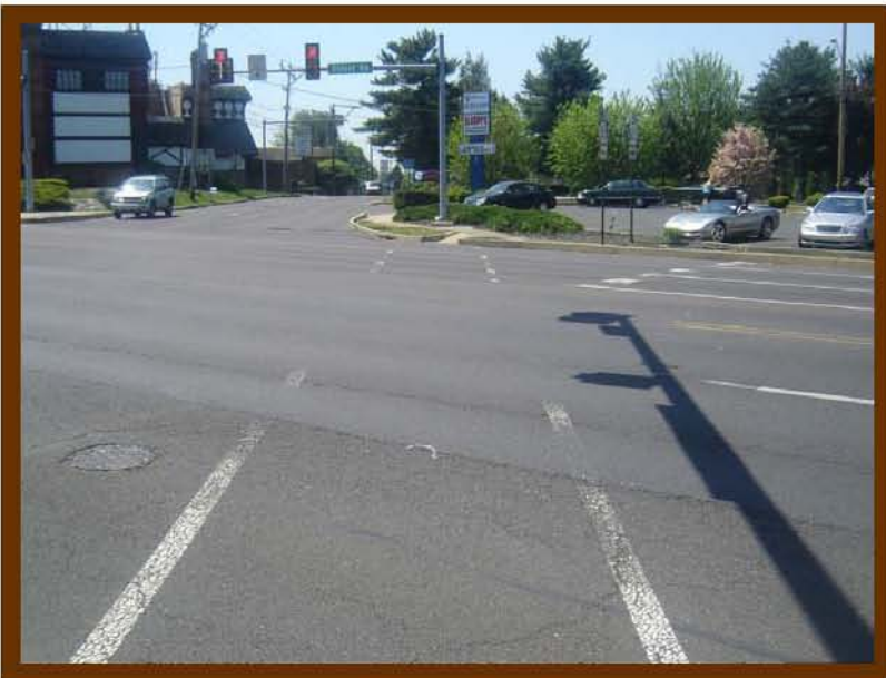
Faded pavement markings at the Hulmeville Road intersection
