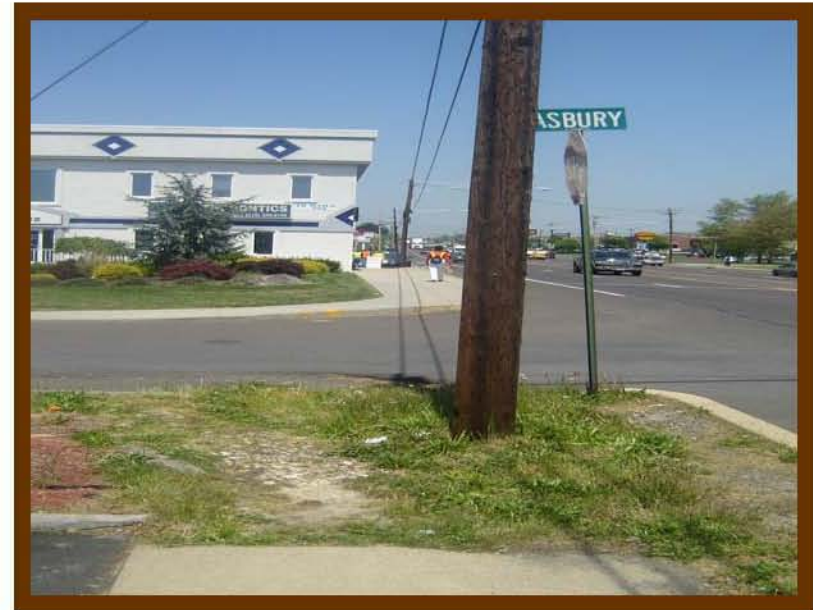
Sidewalk ends abruptly
