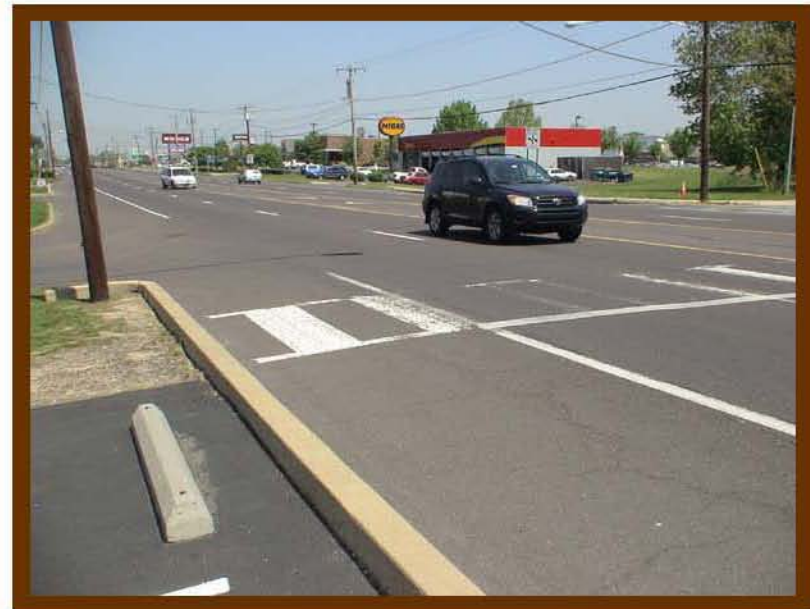
No curb ramp for mid block crosswalk
