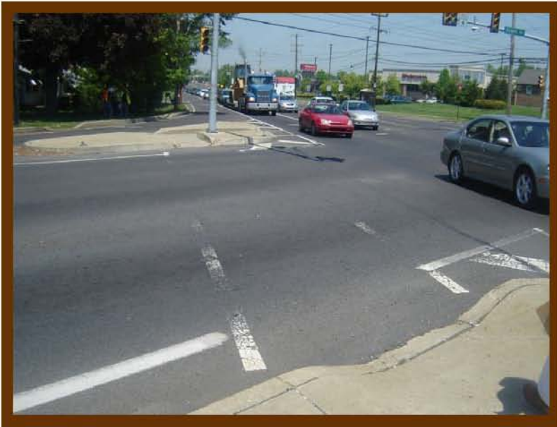
Faded pavement markings at the Knights Road intersection
