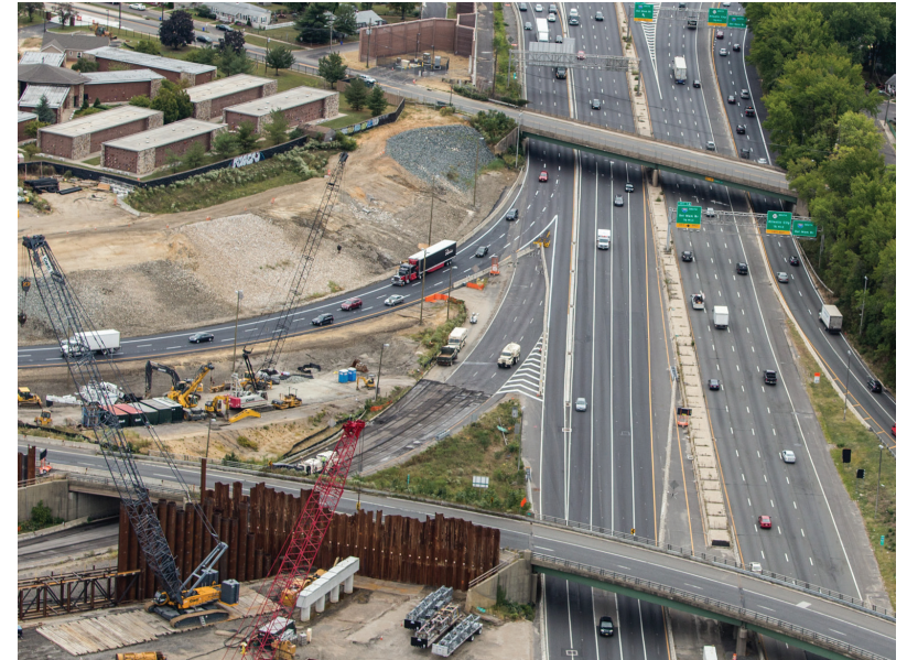
The Route 295/42/I-76 Direct Connection project in Camden County, New Jersey, will provide significant safety and operational benefits when completed. Photo Source: New Jersey Department of Transportation (NJDOT)
