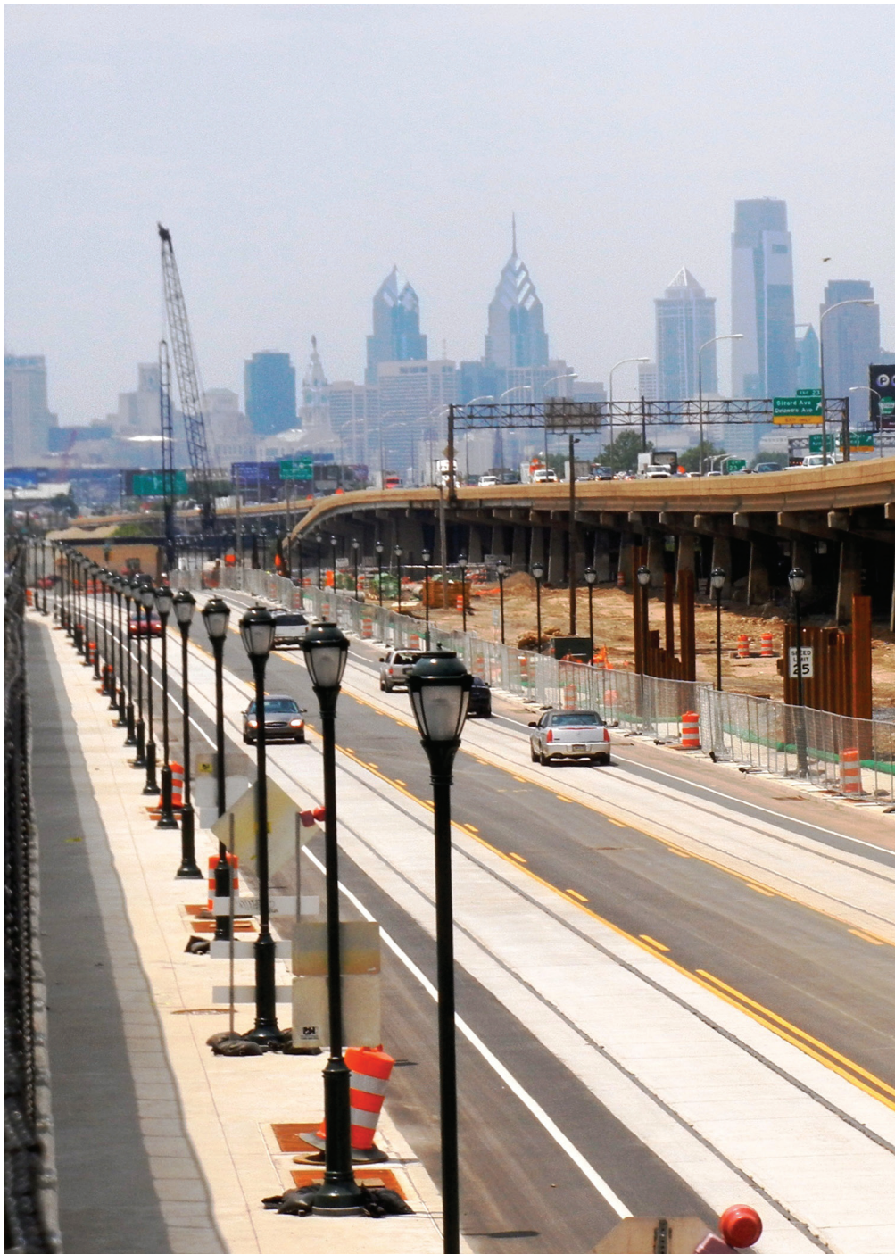
The reconstruction of I-95 in Philadelphia is a multi-year project that includes improvements to the interstate facility, local city streets, transit infrastructure, and amenities for bicyclists and pedestrians. Photo Source: Jim Bergmaier, PennDOT
